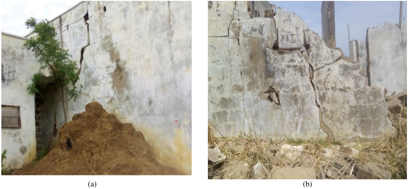
Figure 1. Common structural distress observed in buildings within the study area: (a) cracks on building walls, indicating differential settlement and foundation instability, and (b) dilapidated structures resulting from prolonged structural weakening and inadequate ground support.
